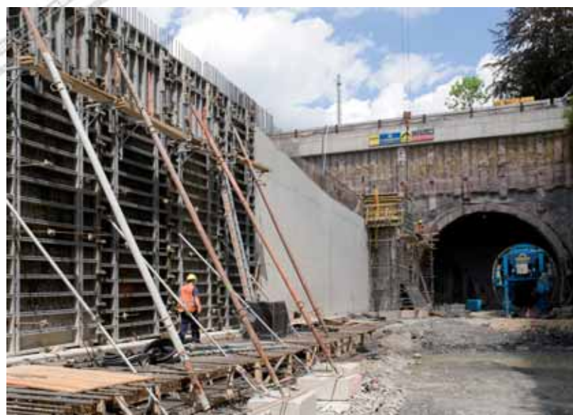
NOEtop large area formwork tables are used for the open retaining wall sections and the cut-and-cover tunnel construction.
