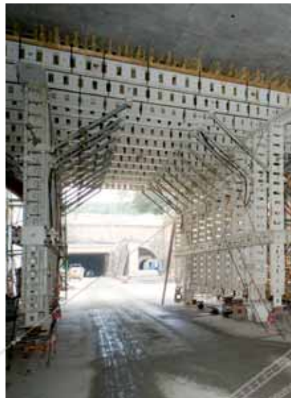
Cut-and-cover tunnel construction west: the NOEtec formwork carriages must allow site vehicles to pass through them to service the rest of the site. Formwork supported by loadbearing towers fills the gap in the area of the road alignment shift.
